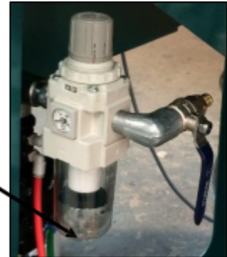
WATER TRAP DRAIN VALVE
